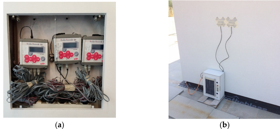
Figure 3. (a) The cavity created in the N-W wall of bedroom 1, hosting the internal dataloggers, and (b) the box powered by a photovoltaic panel, hosting the external dataloggers.
