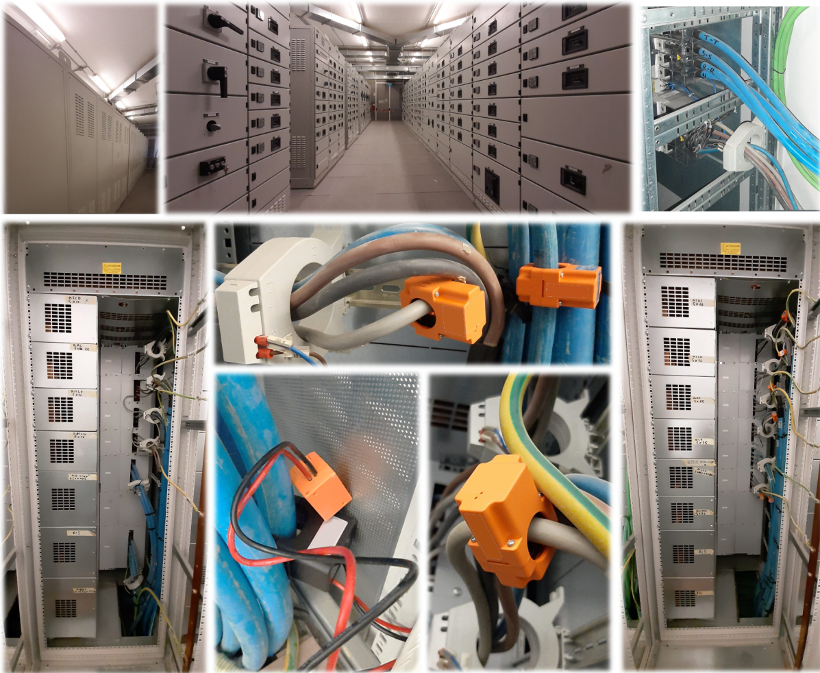
Figure 3.15: Wireless measuring system installed within the building power center
