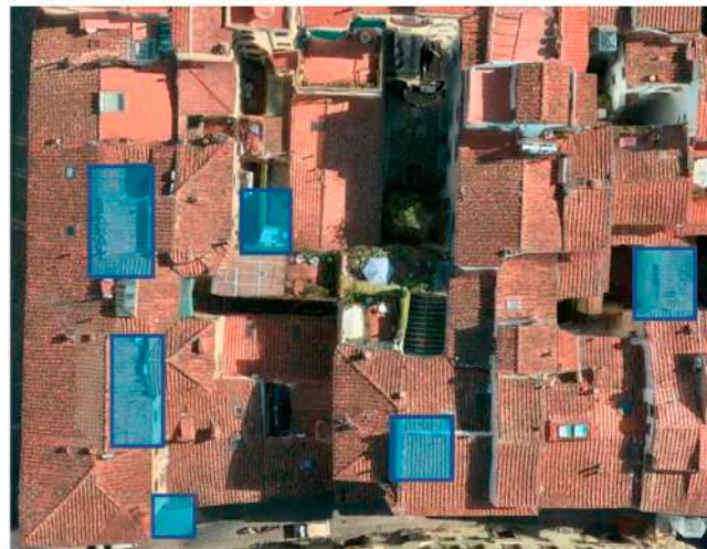
Figure 5. An example of the prospect and roof degradation recognition—blue area: differential degradation.
