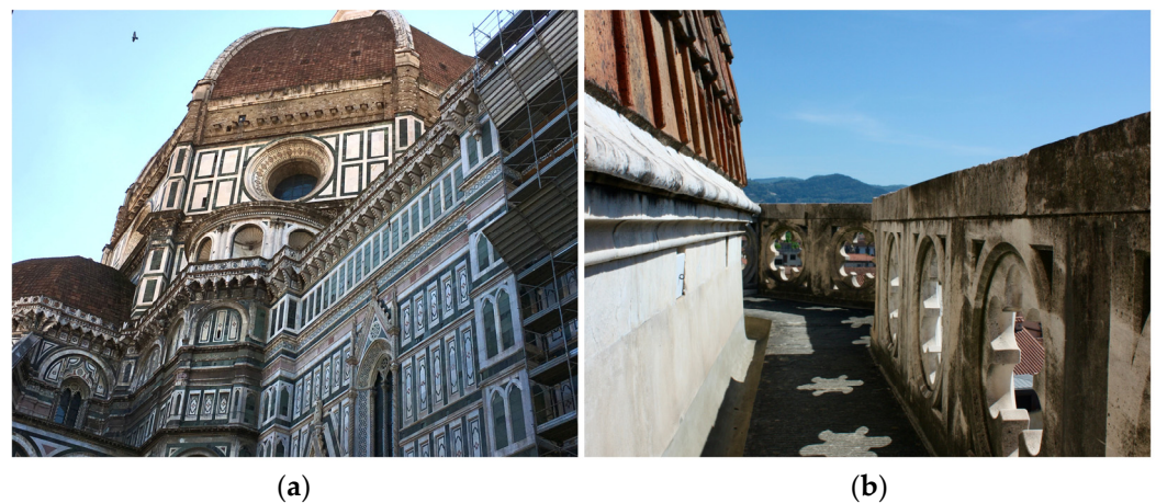
Figure 1. The Cathedral of Santa Maria del Fiore and the study sites. (a) The north-west side of the Cathedral with the external gallery running around the apses. (b) The inside of the openwork parapet of the external gallery at the south-east side, showing a widespread dark patina on marble.
