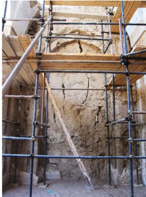
Figure 6 Conservation state of the wall constituting a niche (see online version for colours)
