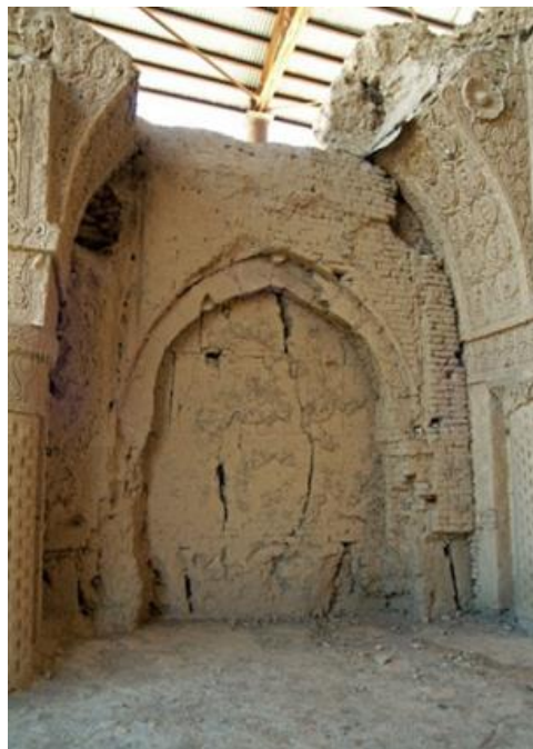
Figure 4 Internal view of South wall, central arch (see online version for colours)
