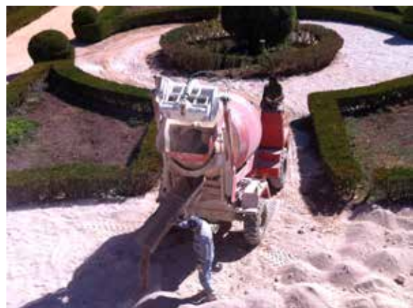
Figure 3. Restoration works at the Botanic Garden of Ajuda (coordinated by landscape architects)
