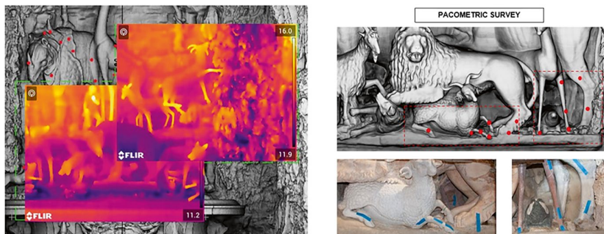
Fig. 11.6 (a) Thermal survey performed on the sculptures; (b) internal reinforcement elements detected by the pacometric measurements
