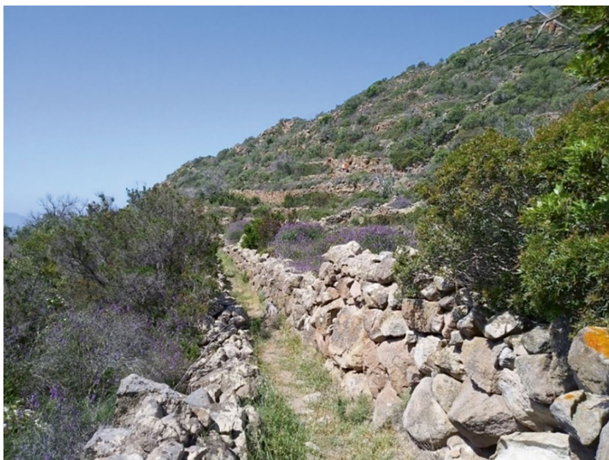
Fig. 17.1 Picture illustrating characteristic dry-stone walls of one terraced area in the island of Panarea (Photo by Alessandro Sardella)
