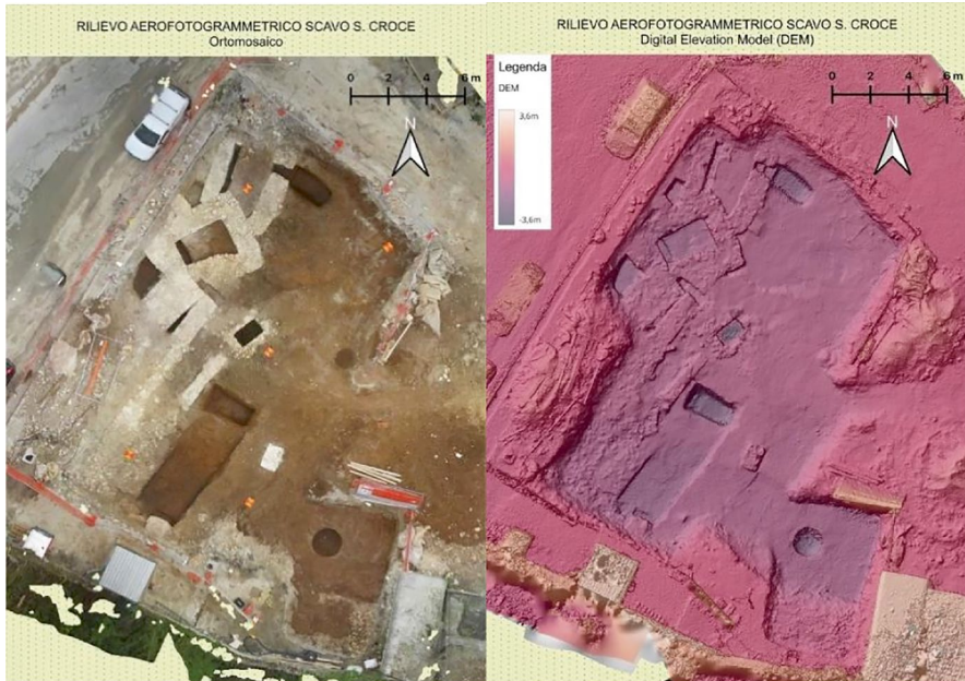
Fig. 3.9 Discovery of structures dating back to the fourteenth–fifteenth century following the demolition of a modern building
