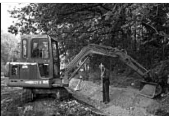
Figure 2. Restoration of loam layer to keep the 'spreng' (manmade water channel) waterproof
