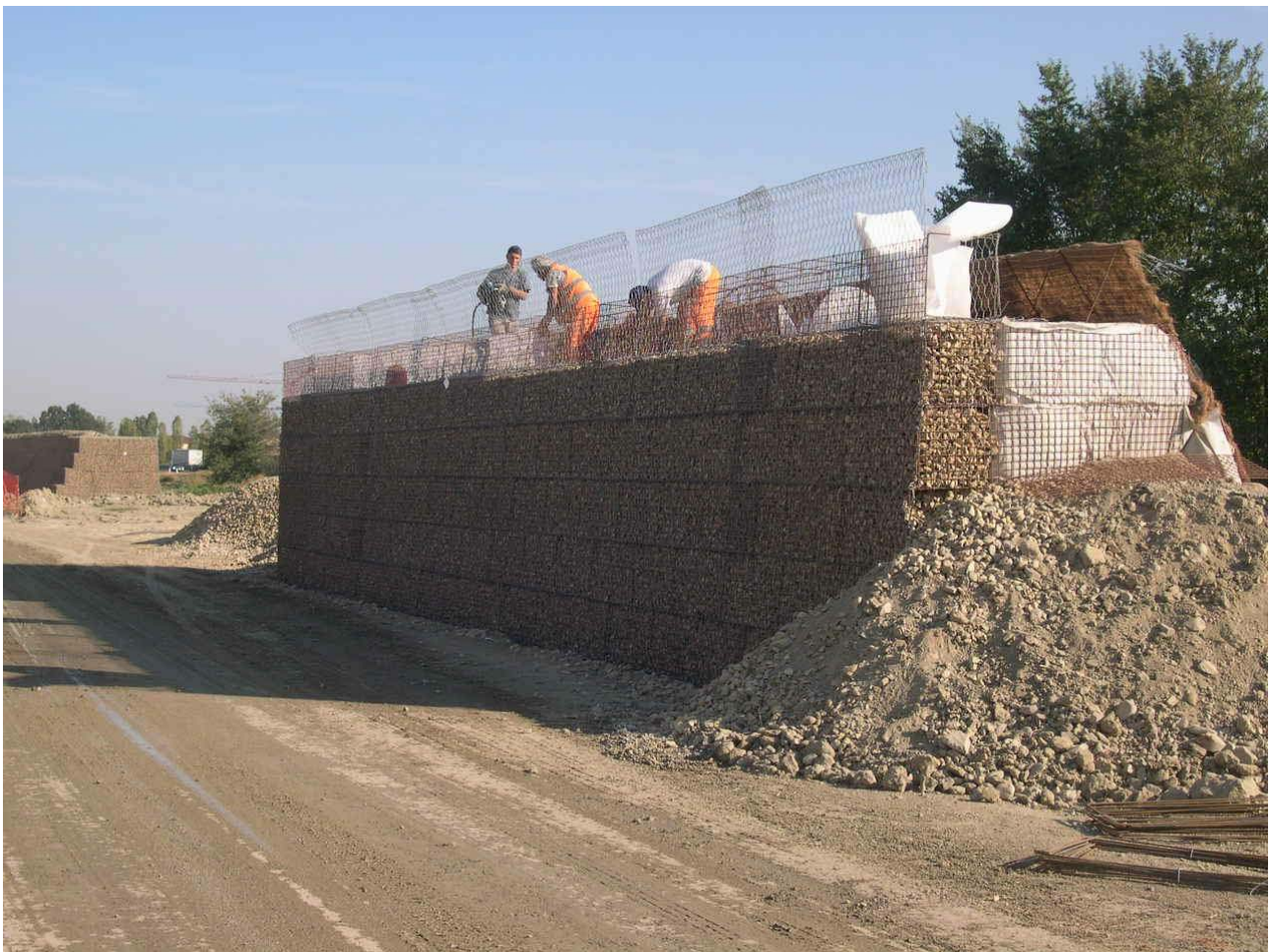
Figure 12 Photo showing the implementation of a test dune, with differentiated 60°/90° slopes, with vertical gabion faces
