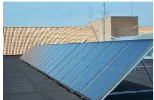
Figure 7 At Aabenraa hospital three solar collector systems were implemented. All the systems were roof mounted. For architectural reasons and in order to avoid glare, solar collectors were mounted so that they aren't visible from outside the building. Special attention was given to the risk of legionella bacteria, by using electrical backup system to ensure that high water temperatures required for avoiding legionella growth were always achieved. Each system includes approximately 50 m 2 solar collectors, which provides an annual energy yield of about 27 MWh per system. This provides about 60% of the annual energy requirement for water heating.
