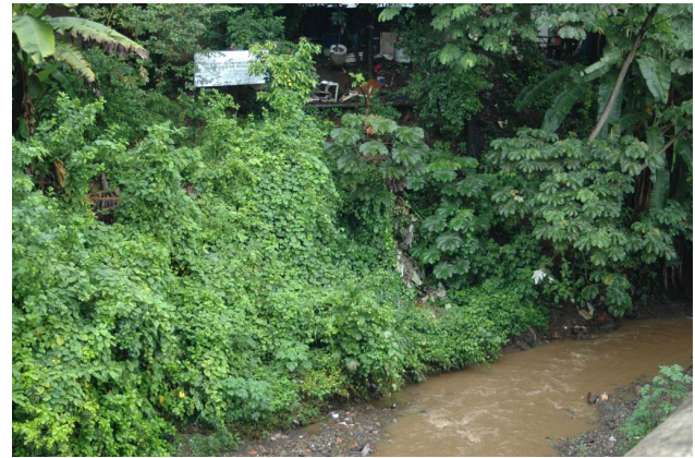
Fig. 10. The riverbank protection (live vegetated crib wall and a slope grating) 44 months after cuttings planted and with sedimentation in the lower part.
