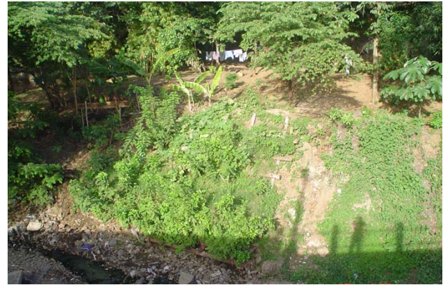
Fig. 8. The riverbank protection (live vegetated crib wall and a slope grating) 7 months after cuttings planted.
