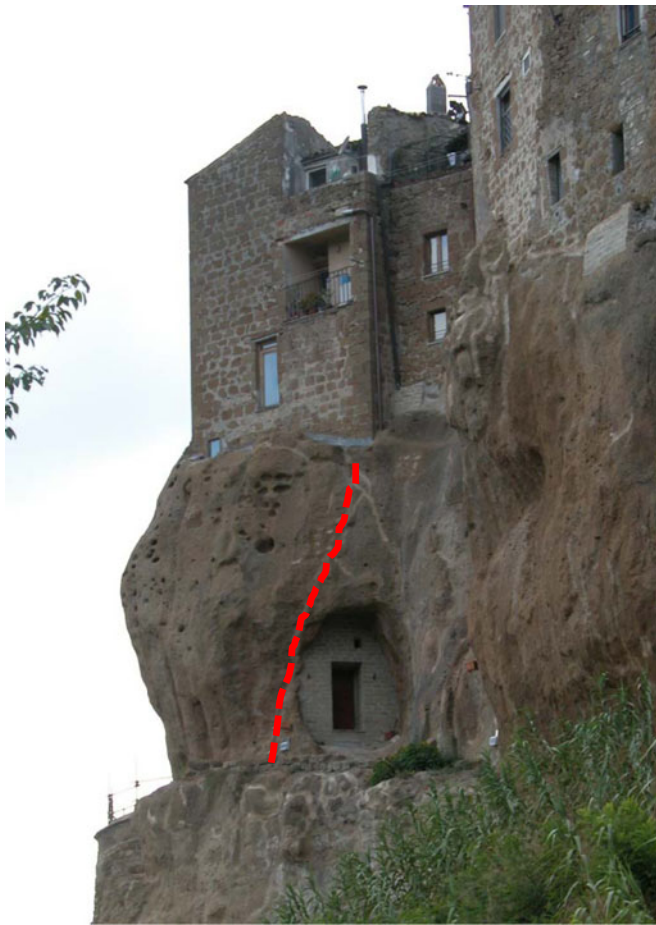
Fig. 14 Test area selected on the southern side of the Pitigliano cliff. Deformometers were installed to monitor the joint ( dashed line ) which controls the wedge geometry. Spatial relationship with the overlying building suggests probable direct impacts on the preservation of the built heritage
