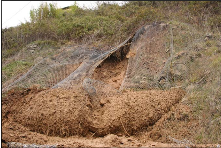
Figure 1.10: one of the Valle Armea landslides occurred in 2000. The landslides has damaged a main road, destroyed a car and injured the occupant.
