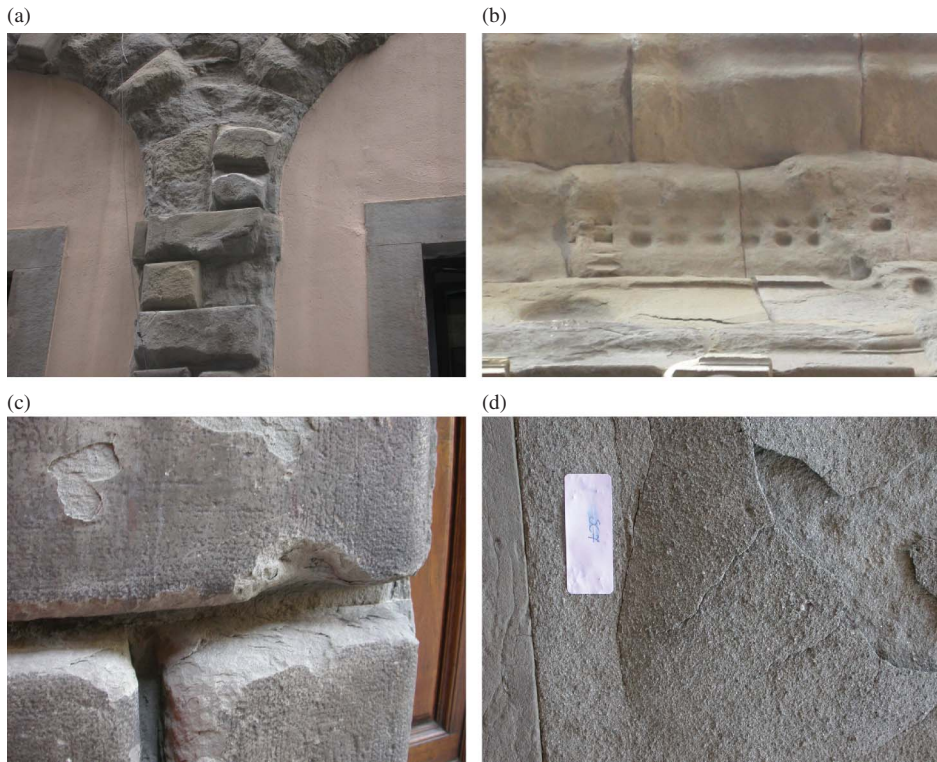
Figure 3. Different decay phenomena at variable scales: erosion, scaling (a), decohesion and dissolution (b), flaking and scaling (c), swelling (d) (color figure available online).
