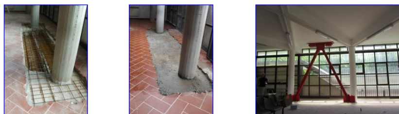
Fig. 19. Construction of the additional R/C beam in one of the two DB alignments parallel to x in the pilotis wing.
