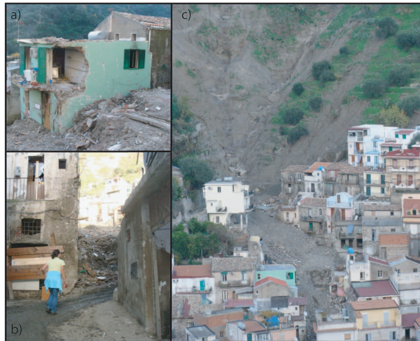
Fig. 4. Examples of the damages caused by one of the seven debris flows that occurred in Giampilieri. In (a) and (b) details of picture (c) are shown.
