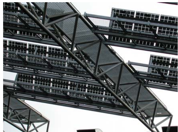
Details of the PV system
