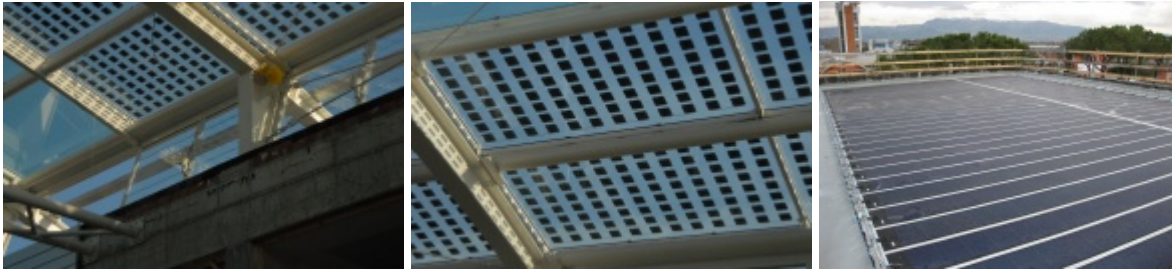
Figure 2. (a,b,) Details of the photovoltaic atrium integrated roof from inside. (c) Detailed of the thin film integration on the roof
