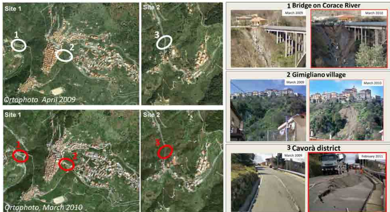
Figure 3. Location and date of recent landslide occurrences in Gimigliano area (1) landslide on the scarp along Corace river, damaging Corace bridge pylons; (2) landslide on metamorphic rocks slope, threatening Gimigliano Superiore buildings; (3) landslide in Cavorà district.
