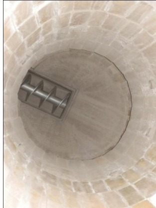
Figure 3-9: Refractory bricks and char extraction screw
