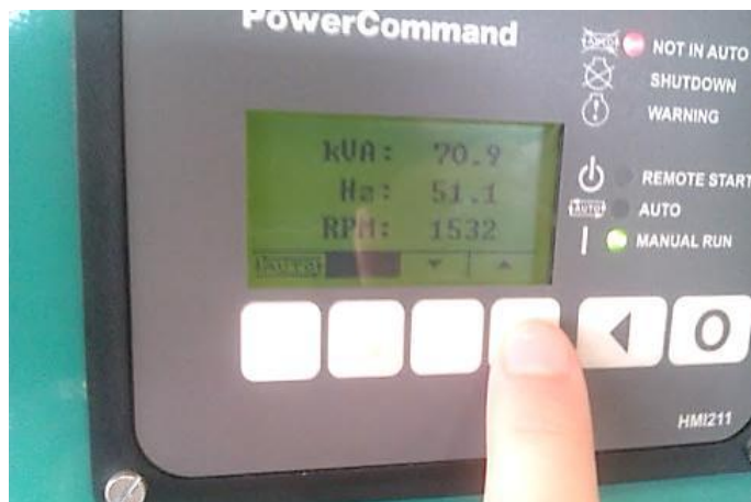
Figure A-16: Engine control panel during full load operation
