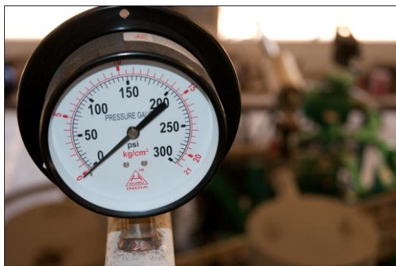
Figure A-11: Pressure gauge in PG line between first and second scrubber
