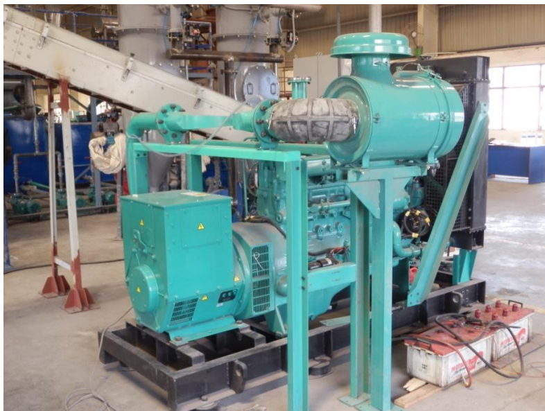
Figure A-10: Cummins G855 70kWe Genset
