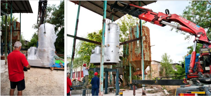
Figure 6-4: Crane elevating reactor for positioning (left). In final configuration the bottom is almost 2 meters above ground level (right)
