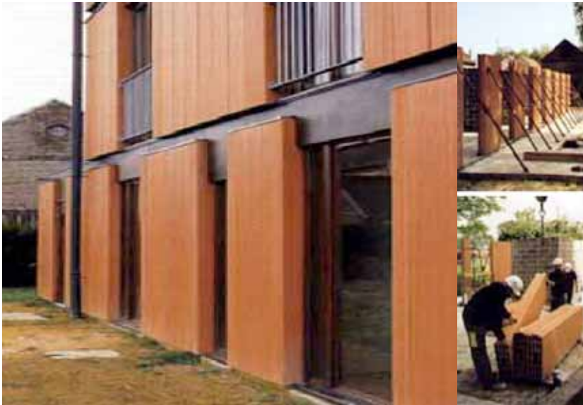
Pic 16- Hotel-management School in Nivillers (F), Tectône, 2000. Construction detail of dry layer facade.
