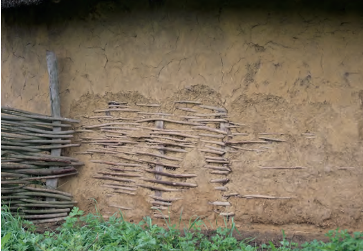
Detail of the exterior walls, Museum Dejbjerg Jernalder, in Skjern. (photos: Jacob Merten) Construction site for compressed earth blocks (CEB), by OSKAM company, in Kolind.
