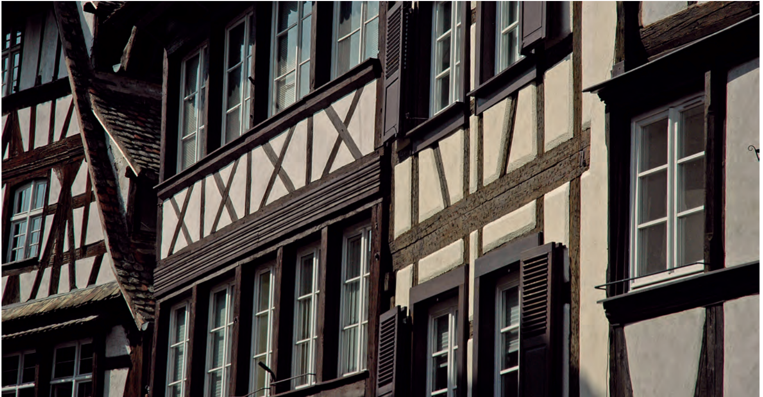
Timber-framed houses, formerly filled with wattle and daub, now with current materials: bricks or cellular concrete, Alsace, France. (photo from Terra Incognita. Discovering/Preserving European earthen architecture , Argumentum/Culture Lab Editions, 2008)
