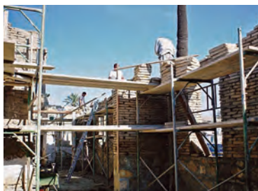
Use of adobe bricks in the restoration of the Museums of the Pancyprian Gymnasium, Nicosia, Cyprus.
