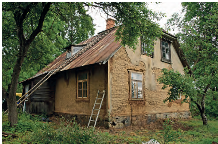
Rammed earth dwelling house built in 1926. The facade after the removal of damaged parts of the old plaster. Rēzekne district, Viļāni parish. (photos P. Blūms)
