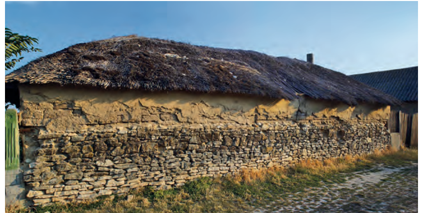
Abandoned traditional house in Jurilovca. (photos: Cătălin Berescu)
