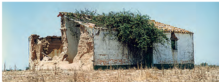
House in Vale da Eira, Santiago do Cacém, south of Portugal. (photo: Mariana Correia)
