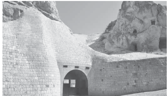
Fig. 29-30 Toakali Kilise and the Church of S. Barbara in Goreme. Examples of wrong conservation interventions.
