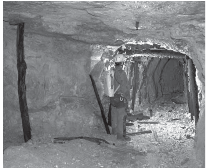
Fig. 5 The supporting structure for the vault in a bauxite mine (Cusano Mutri, Monti del Matese - Campania) is realized in correspondence with a karstic fracture (photo: N. Russo). The drip of the drainage through the same fracture is evident.
