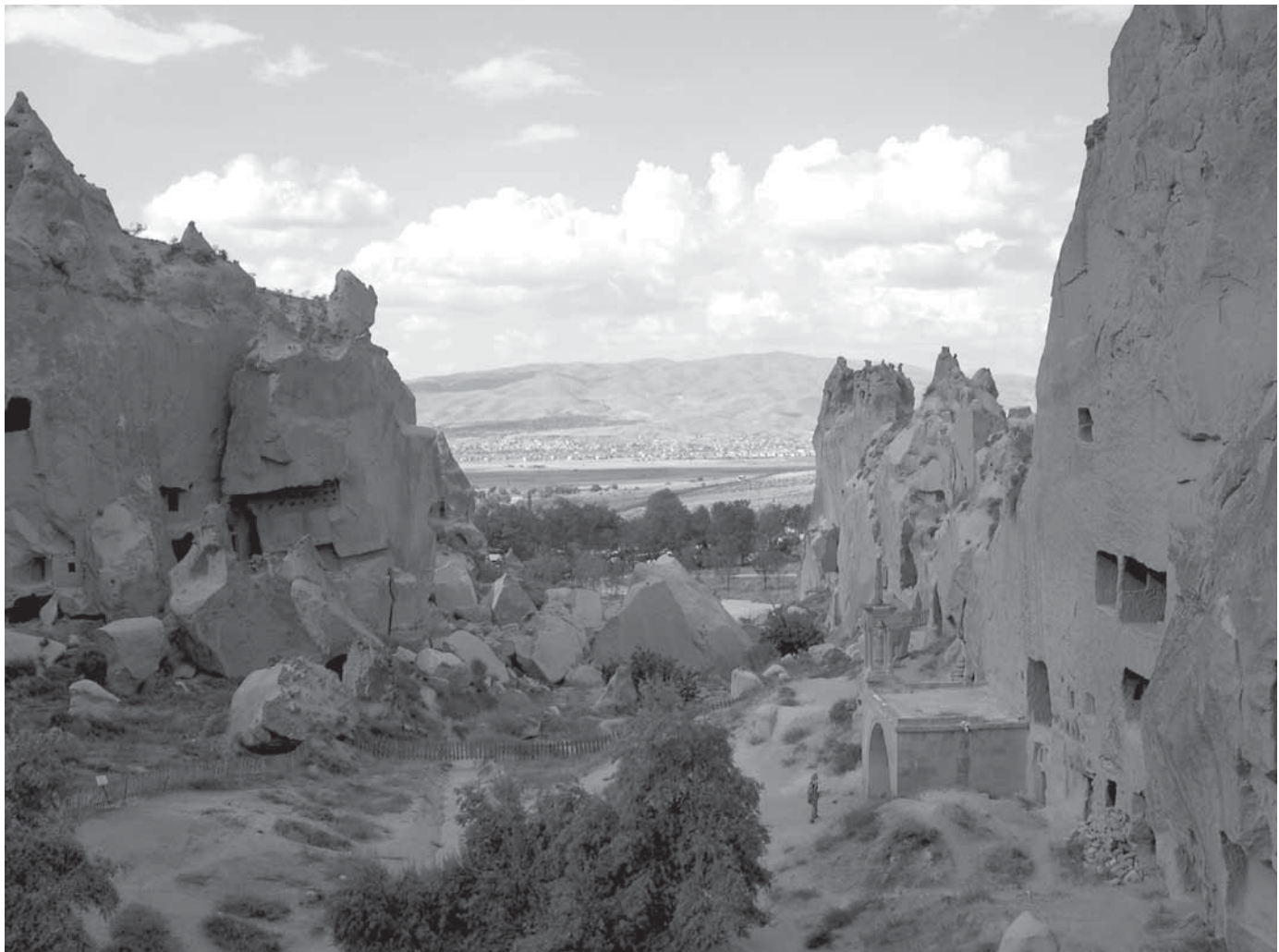
Fig. 19 Zelve. The wide de-tensioning fracture on the tuff cliff has revealed the underground rooms (photo: R. Bixio, Centro Studi Sotterranee). The evolution of the fracture will cause the collapse of this side of the cliff.
