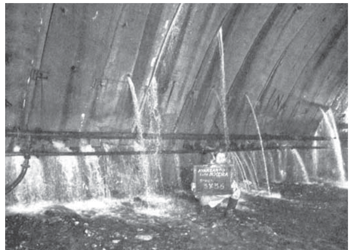
Fig. 6 Floods during the works for a railway tunnel, Nocera - Salerno (from Celico et al., 1977).
