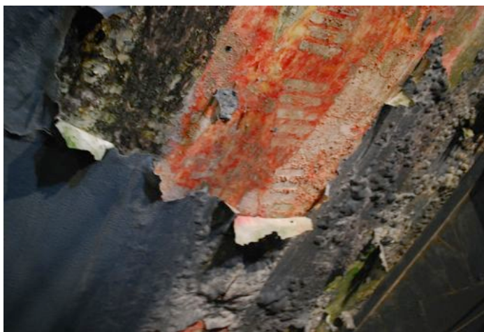
Figure 8.2. The water infiltration that caused the detachment of the complete section of overpainting paint film, revealing the original paint of Capogrossi . The detached paint fragments were used for the cleaning tests carried out in laboratory.
