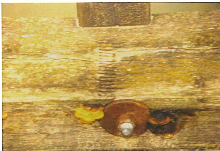
Figure 1: Timber-bridge n. 9. Fruiting bodies of brown-rot fungi, close to moisture trap (hole, bolt and washer).
