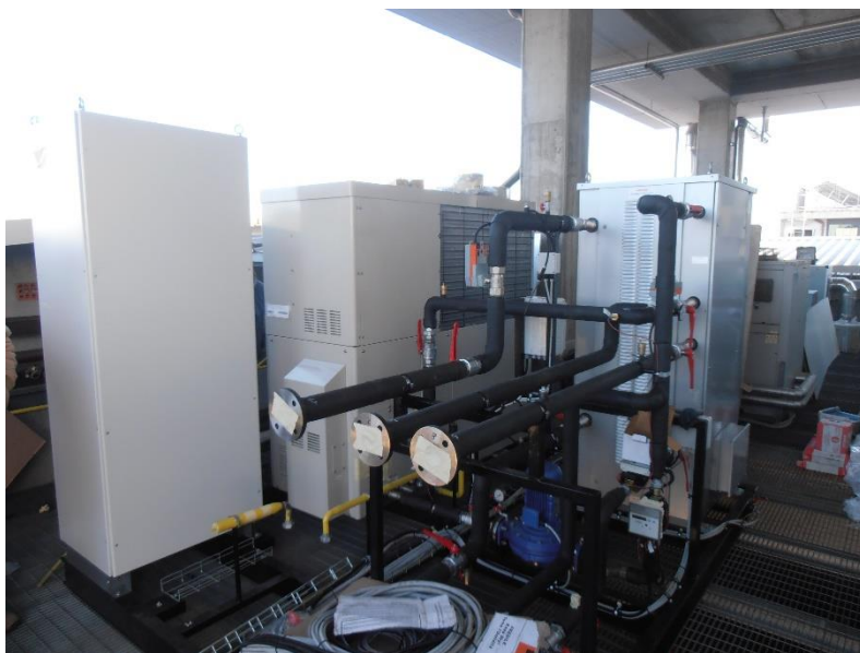
Figure 11 - Skid assembly on Pontlab terrace
