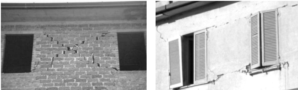
Figure 54: On the left, diagonal cracking; on the right, bending cracking. (Theoretical manual of 3MURI)
