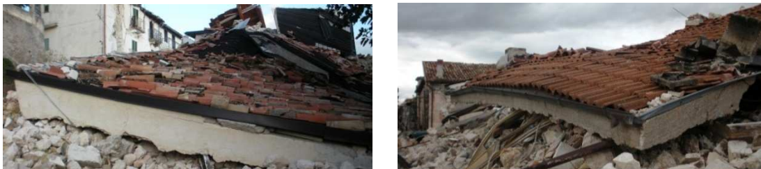
Figure 18: Two collapsed heavy roofs in Castelnuovo (AQ).
