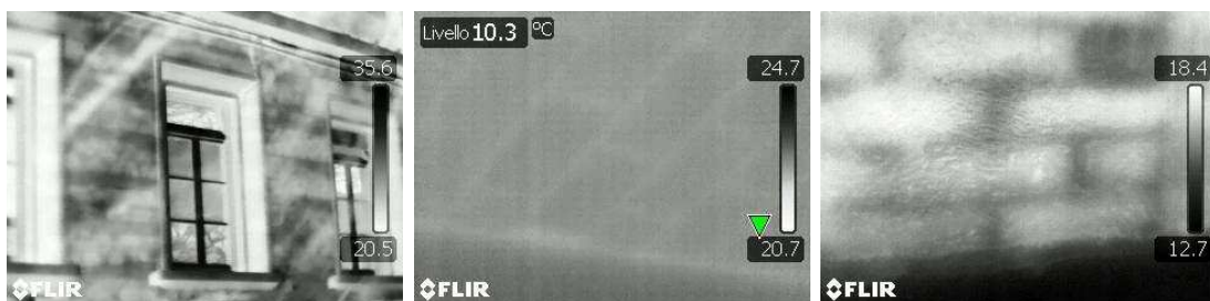
Figure 43: Thermal images: (left) stone masonry with brick layers, (middle) reinforced concrete floor, (right) brick masonry.
