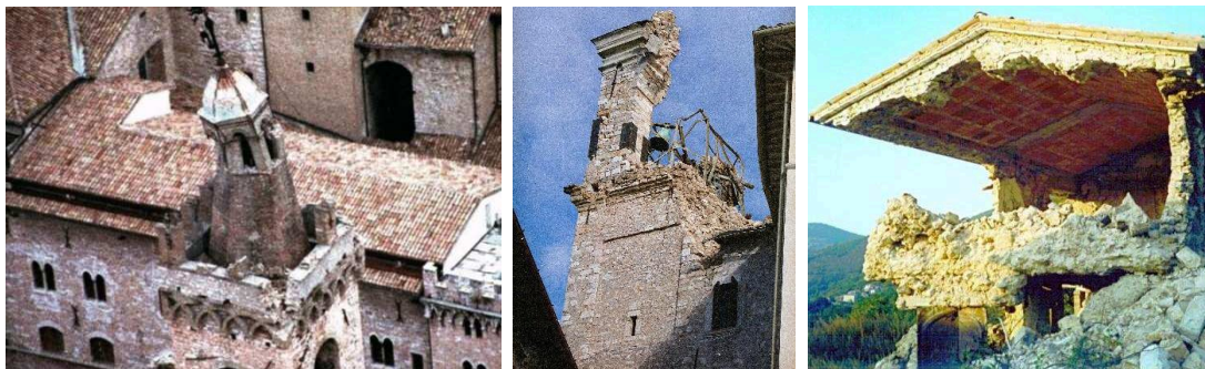
Figure 5: The Cathedral of Foligno before the collapse of the Bell-Tower (left), the Historical Tower of Nocera Umbra (middle) and a particular collapse for a restored building with a reinforced concrete roof (right).
