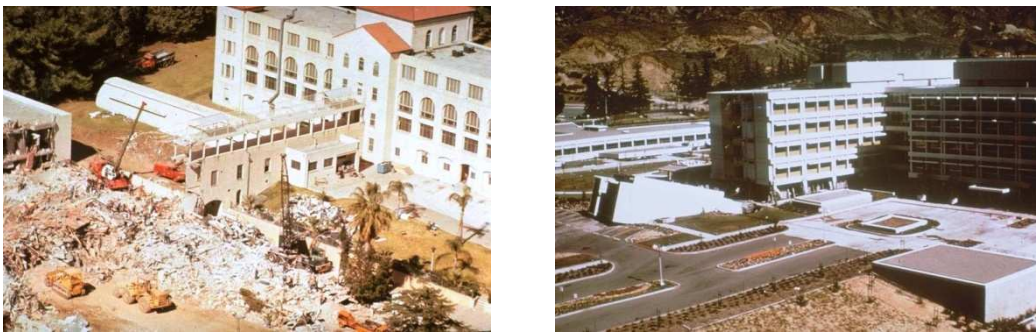
Figure 45: Damages to the San Fernando Veterans Administration Hospital, built in 1926, before the development of earthquake building codes (left). Damages to the Medical Treatment and Care Building (Olive View Hospital complex), completed in 1970: the first storey has nearly collapsed and the towers containing the stairs (structurally separated from the building) have overturned (right).
