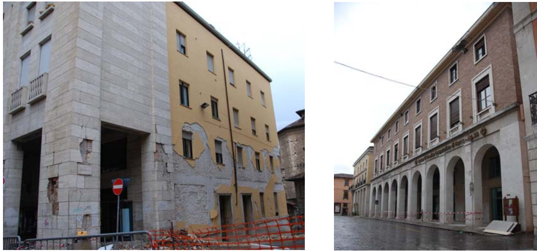
Figure 1. Public buildings of the 30s in L'Aquila (central Italy) affected by the earthquake of April 6, 2009.
