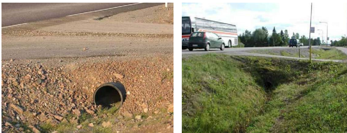
Figure 55: Examples of hazardous drainage features (Source: [A.2])
