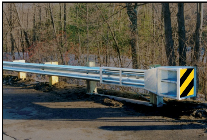
Figure 11: A Midwest non-proprietary energy-absorption terminal
