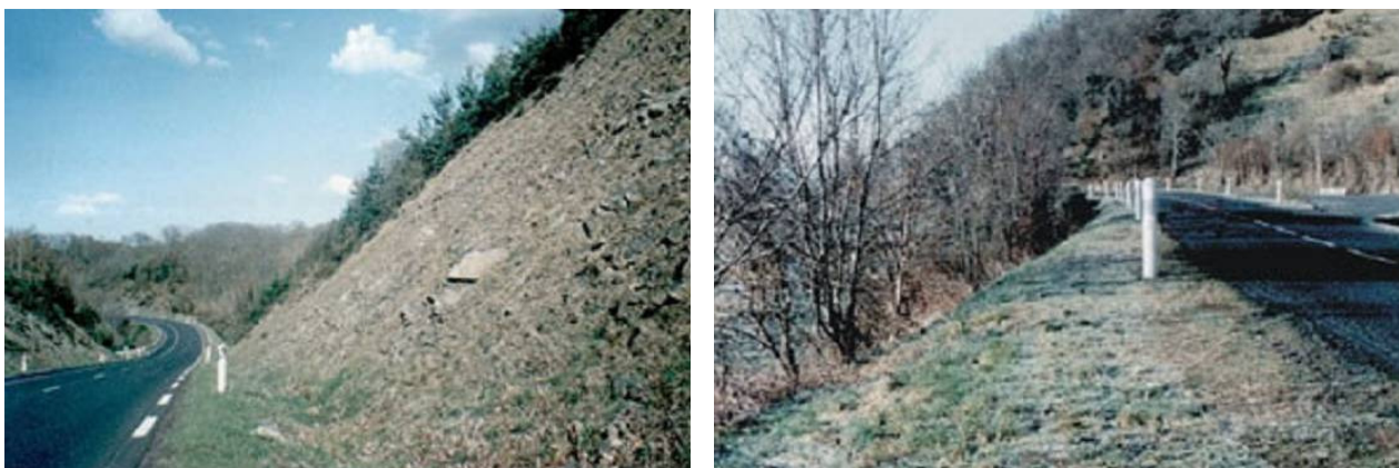
Figure 56: Examples of hazardous cut ( left ) and fill slopes ( right ) (Source: [A.2])
