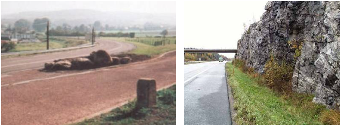
Figure 54: Examples of hazardous boulders ( left ) and rocks ( right ) on the roadside (Source: [A.2] and [A.3])
