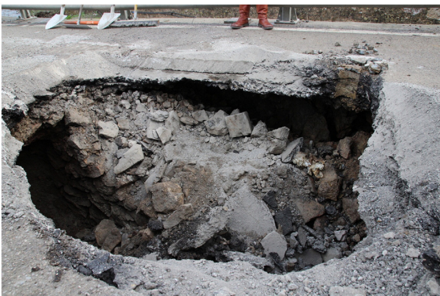
Fig. 7. Photo of the cavity below the PR26C detected by the GB-InSAR on 4 February 2014.
