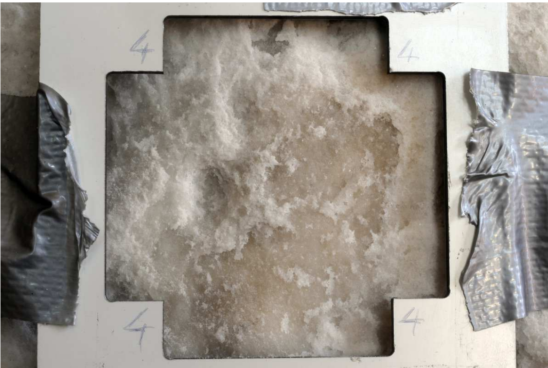
Fig. 7 – Marble from the spolia of a Roman column placed in the basilica during the Romanesque period. This stone shows evident surface alteration with strong decohesion and fine exfoliation (Copyright Stefano Columbu and Giorgio Verdiani).
