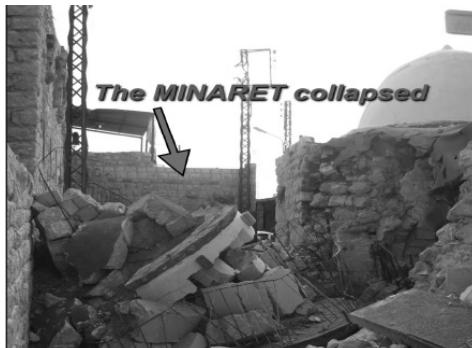
Fig. 3 Chama mosque: the collapsed minaret.
