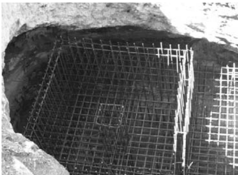
Fig. 4 Chama mosque: the ancient cistern (probably dating to the Roman period) about to be filled with reinforced concrete.
