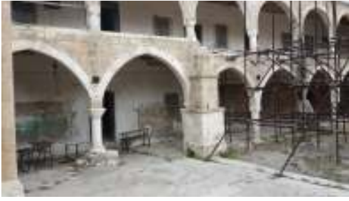
Figure 8 – The scaffolding is holding in place the leaning column, urgent intervention is required (photo: A. Camiz, 2014).
