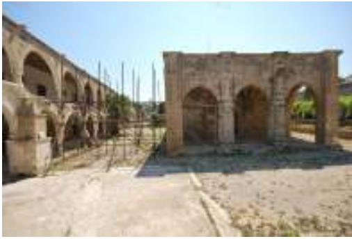
Figure 9 – The scaffolding is holding in place the leaning column, urgent intervention is required (photo: A. Camiz, 2014).
