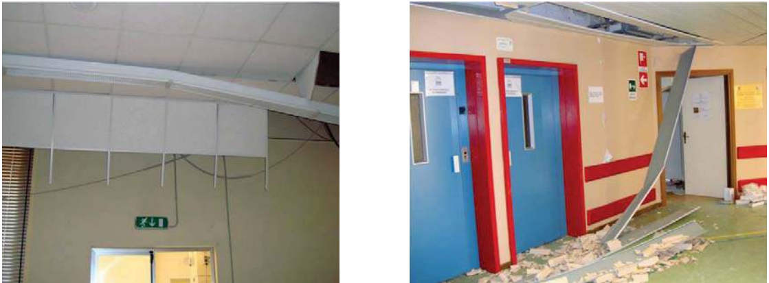
Figure 1.5 Damage to the ceiling during the l’Aquila Earthquake.
