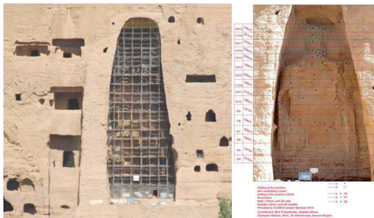
Fig. 4. The scaffolding for the stabilization of back wall shear zone and the position and typology of installed anchors (diam. 22mm, 12mm, 6mm)
