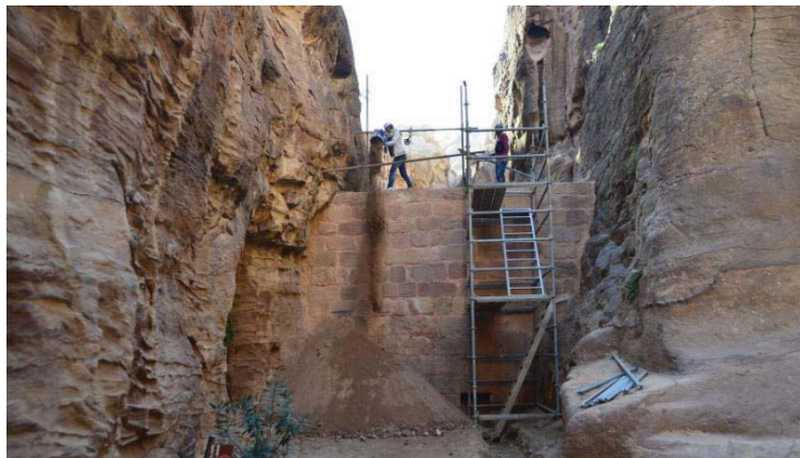
Fig. 6. Manual and proper cleaning of stone dams, to protect the Siq of Petra from flash flood.
