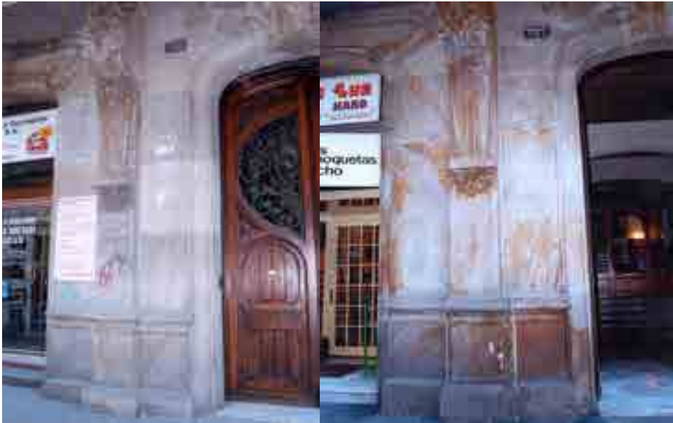
Fig. 4- Case study of anthropic weathering of Montjuic sandstone (Mallorca Street 325-327, Barcelona). The left picture shows the façane prior to cleaning, while on the right we can note the effects on several blocks of the poorest quality variety of Montjuic sandstone (the so-called “rebuig”) with red staining related to oxidation of the iron-rich cements of the rock, while other blocks of the best quality (“blancatge” variety) show excellent preservation of the original color of the rock. This kind of alteration is enhanced when the cleaning is conducted with water-acid jet beam, and till know is retained irreversible.
