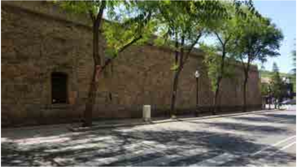
Fig. 7 - Outer wall of the Baluard of Drassanes (Bastion at the medieval wall of the city of Barcelona, conserved at the sea side of the city attached to the former dockyards, now Museu Marítim and municipality dependences). All this protective wall of the open port of Barcelona is built with Montjuïc sandstone, as well as the XVI century dockyard). Most of the medieval walls of the city were removed during the metropolitan expansion of the city during the second half of XIX century, being now just preserved at the Drassanes site and in the north opposite side of the city in some inner dependences of the Ciutadella Castle, built after the Catalanian defeat in Spanish Succession War (1714).
