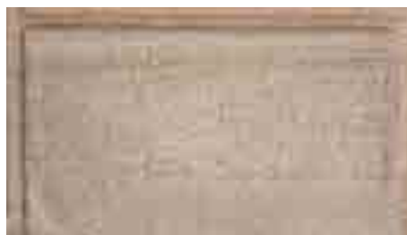
Fig. 1- Typical macroscopic feature of the Montjuïc Sandstone, including moderate evidence of lamination and cross-bedding after diagenetic lithification and pervasive silicicementation (façade of Passatge de la Pau, Barcelona).
