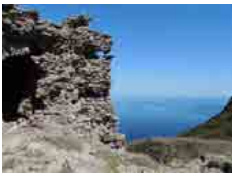
Fig.7 - Tower of Barbici: the deeply eroded masonry.
