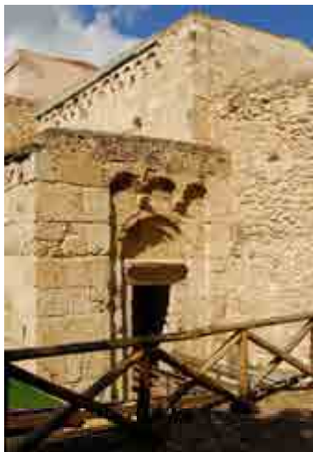
Fig. 1- San Saturnino Church (Cagliari, south Sardinia). The photo shows part of Romanesque masonry constructed with ashlars of Pietra Cantone limestone (similar to Pietra di Lecce) with decay macroscopic forms.
