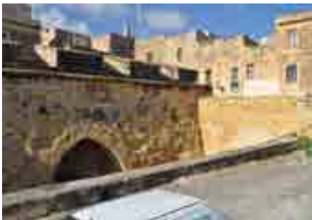
Fig. 8- Birgu, Malta. Scaling and back weathering on southern fronts (M.Acierno 2011).
