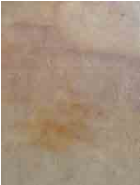
Fig. 2- Typical macroscopic feature of the Montjuïc Sandstone, including moderate evidence of lamination enhanced by the presence of Fe-rich minerals. Note the fade of oxidation, a common feature in this rock when it has undergone severe acid cleaning (façade of Passatge de la Pau street, Barri Gòtic, Barcelona).
