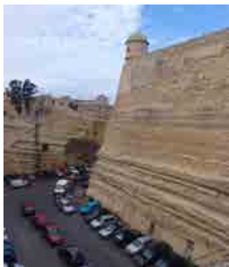
Fig. 7- Valletta, Malta. Rock bench and masonry degradation (Marta Acierno 2011).
