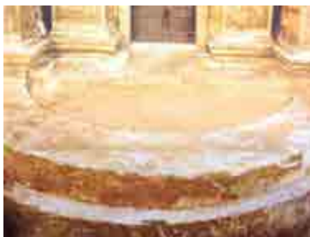
Fig. 1- Foundations of the stronghold in the northern front of the Cathedral of Almería (Ana Pérez, 1998).
