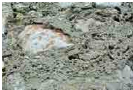
Fig. 7- Weathering of plaster.
