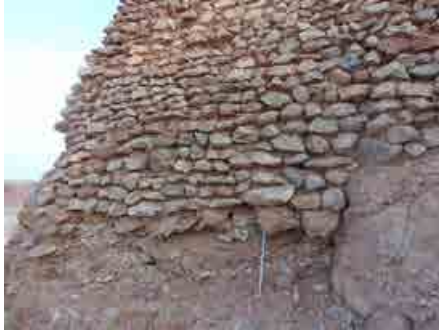
Fig.3- Aghem of Taguelzi. Constructive detail of the stone boundary walls (Illili Mahrour, 2015).
