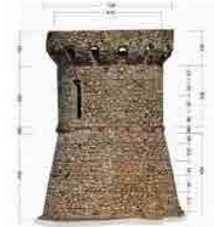
Fig. 10- Tower of the Isolella, survey of the mass volume with the photogrammetry program Autodesk 123D Catch (Casu, Pisu, 2013).
