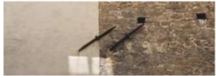
Figure 5. Anchor plates connecting two adjacent buildings in Florence, Italy (credits: L. Dipasquale).
