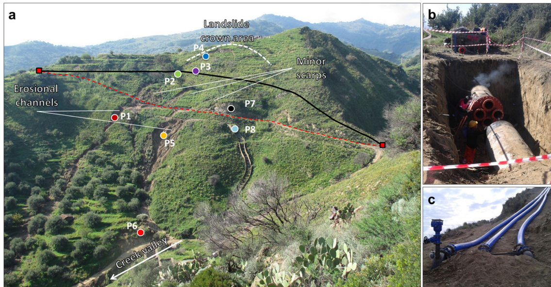
Fig. 3 a Image of the Calatabiano landslide acquired on 10 November 2015, from the monitoring system installation point. The dashed white line represents the main landslide crown, the dashed red line represents the interrupted pipeline (b), and the black line represents the new pipeline by-pass (c). P1–P8 represent the GB-InSAR monitoring points
