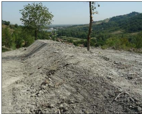
Fig. 52. Earth-fill dam, built during safetying operations in landslide area (the position is shown in Fig. 51).
