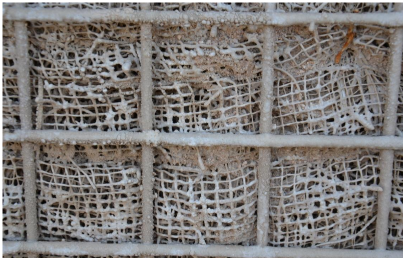
Figure 1-18 Effect of dust and salt water on the pad material (Southern Iraq).
