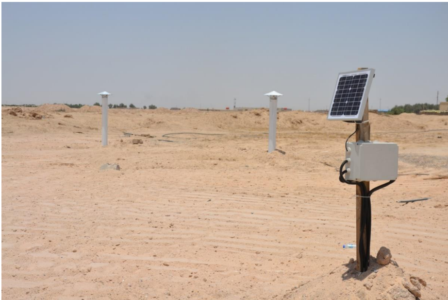
Figure 2-11 The beginning of the operation phase of the earth-to-air heat exchangers system.
