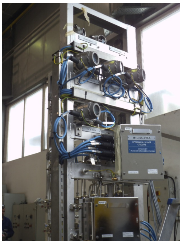
Figure 3.16: Transmitters installed on the physical plant.
