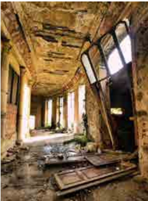
Fig. 29 - Lateral passage in serious decay inside the Corallo Baths (G. Verdiani, 2012).
