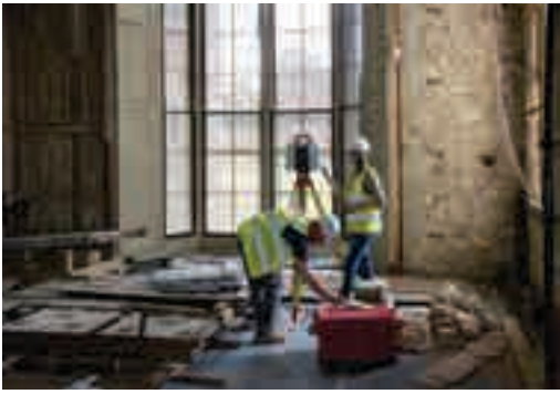
Fig. 4 - Laser scanning of Ballroom during enabling works: removed panelling can be seen stored on the floor and exposed stonework of late medieval solar walls (© MOLA)
