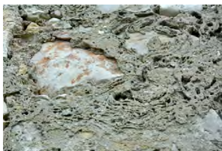
Fig. 7- Weathering of plaster.
