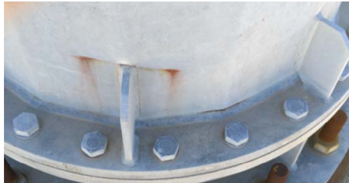
Figure 1. Fatigue damage to the steel supporting pole of a 20kW horizontal axis wind turbine
