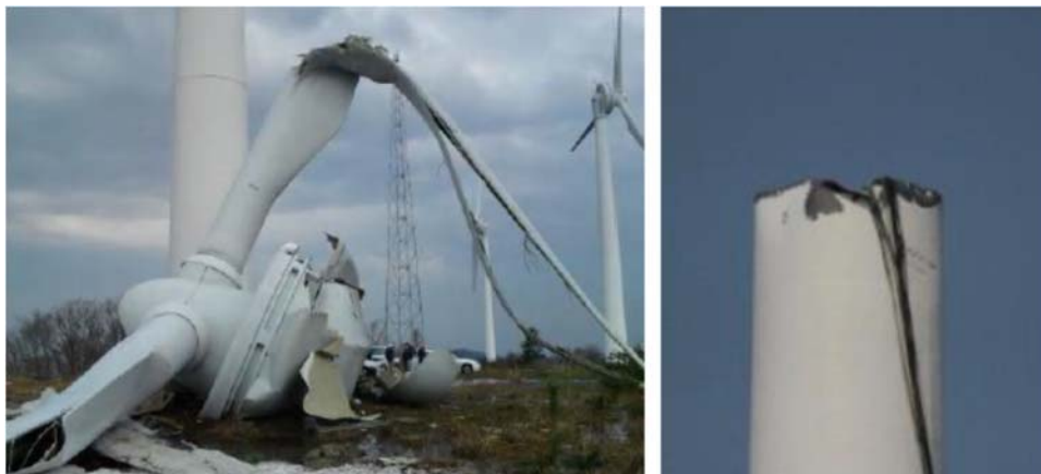
Figure 1. Accident in the Taikoyama wind power plant caused by a fatigue failure [3].
