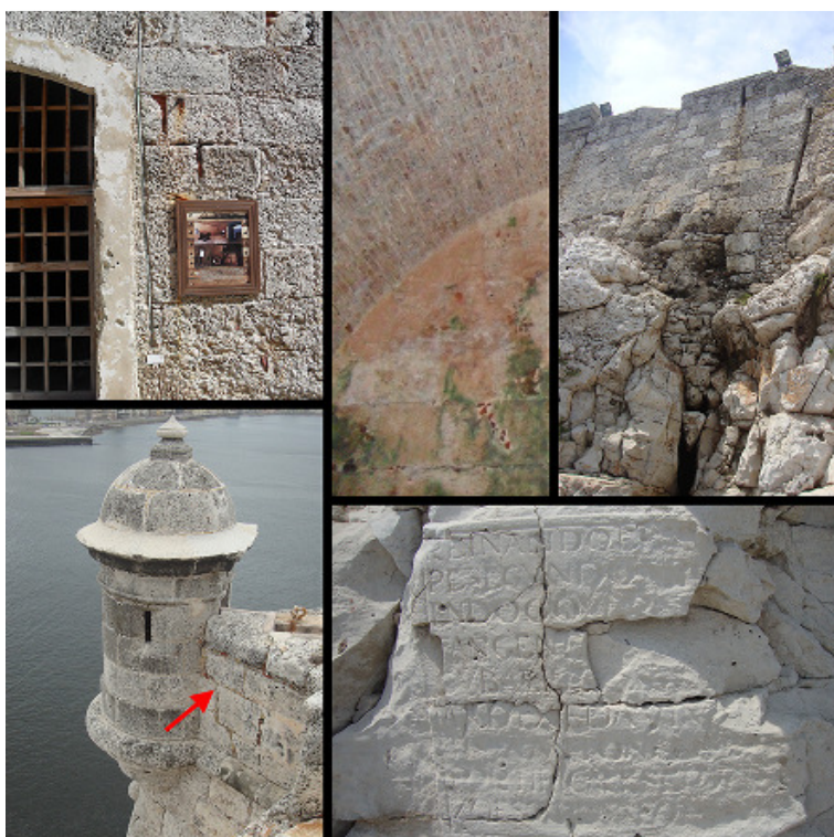
Figure 3 – Some current emergencies of degradation by various causes: environmental, material and structural deterioration
