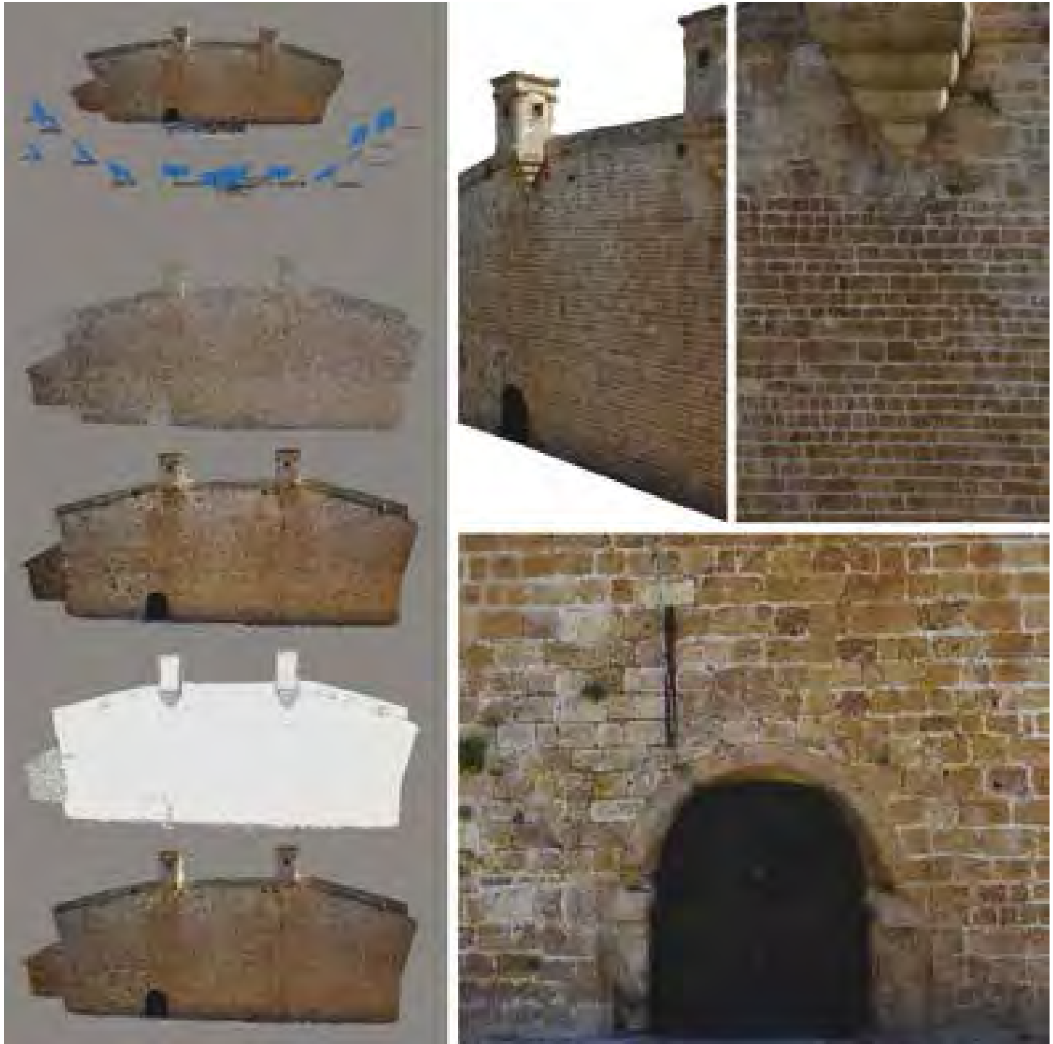
Photogrammetric survey of a part of the eastern city walls of Acre (rebuilt in the XVIII century). On the left side the acquisition process with the placement of the camera and the reconstruction process of three-dimensional model of the photographs sequence. From top the sparse cloud, a dense mesh model without textures and the final model with the application of textures. On the right, some details of the model with texture.
