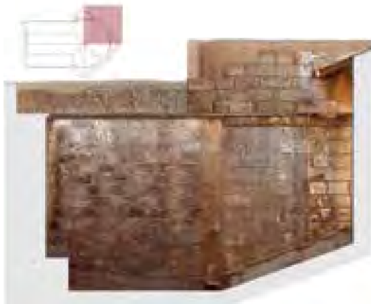
2d vectorial drawing and photo mosaic of the North Corner, east side. As per the upper pictures, in this case the state of conservation can be evaluated. The chromatic alteration is due to the microbiological attack and to the rain-water action.
