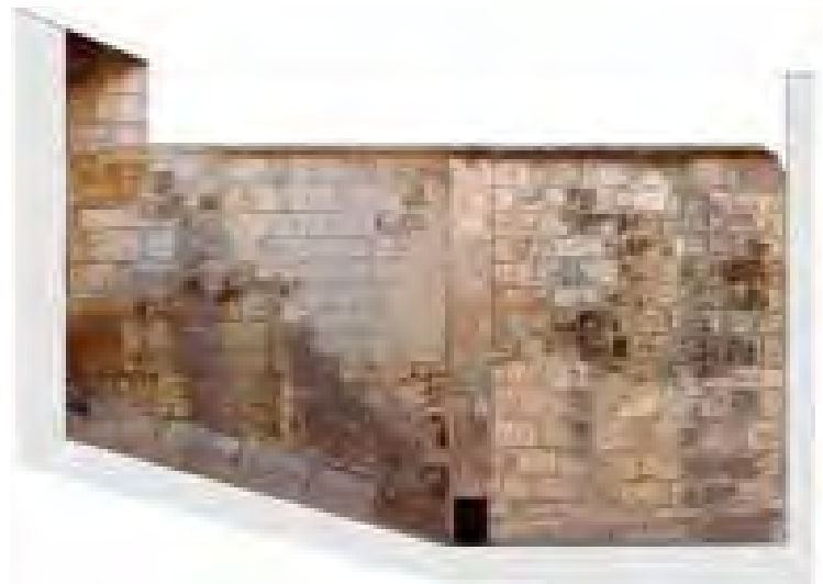
2d vectorial drawing and photo mosaic of the North Corner, north side. In this case the state of conservation can be evaluated. On the left side shows a whole area of loss stones, filling with concrete material.
