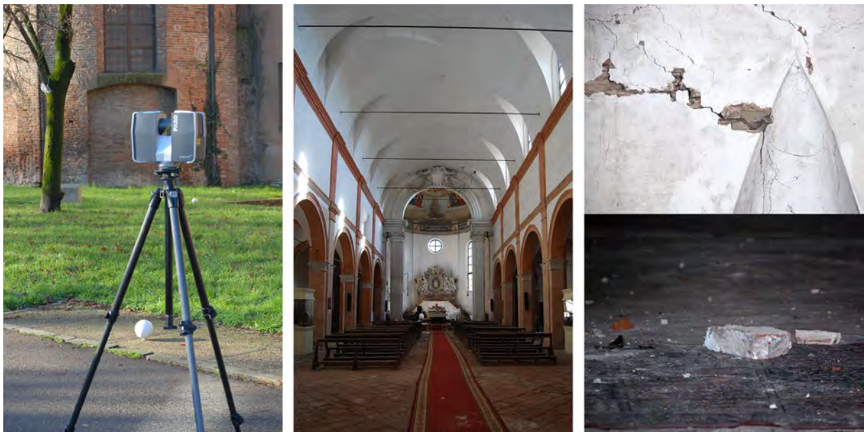
Fig. 3: The church of Santa Maria della Consolazione in Ferrara. From left: the laser scan station Faro Focus 3D used for the digital survey; the nave during the surveying operations; part of the vault collapsed in the earthquake.
