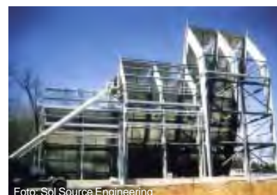
Foto: Sol Source Engineering
