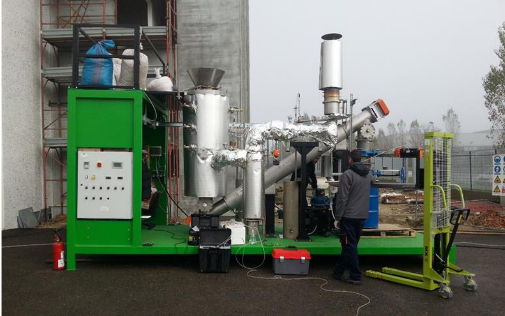
Figure 44. Carbonization unit during functional test operations
