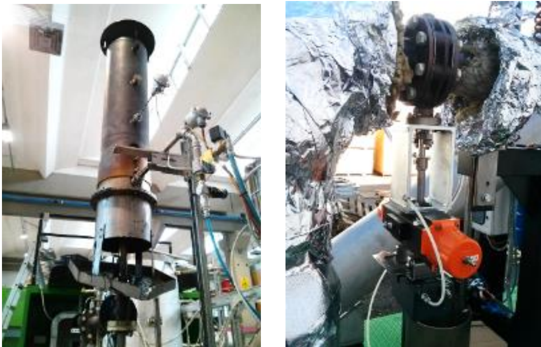
Figure 39. Details of stack and gas regulation valve
