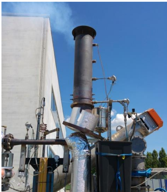
Figure 64. Exhaust gas sampling point at stack
