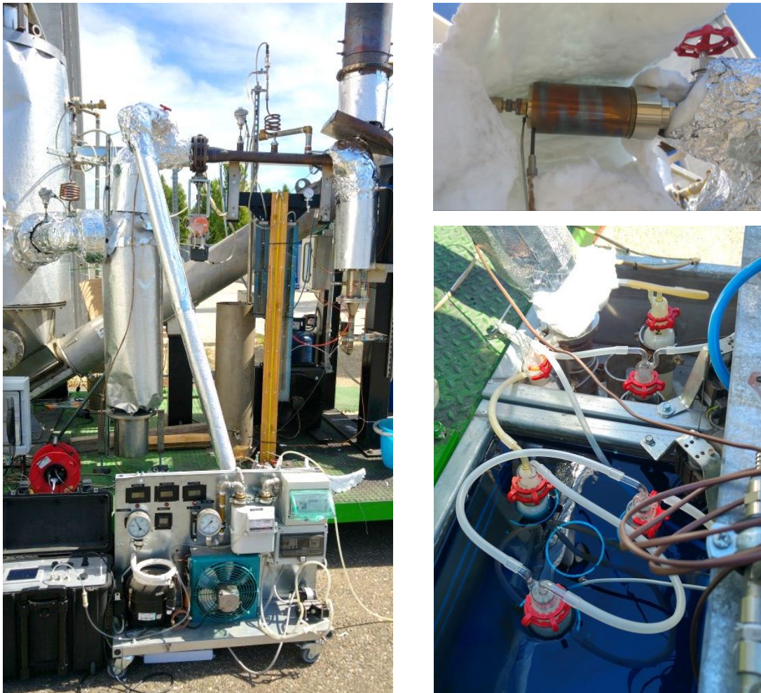
Figure 63. Tar sampling installation details: thermostatic line and filter, impingers bottles configuration
